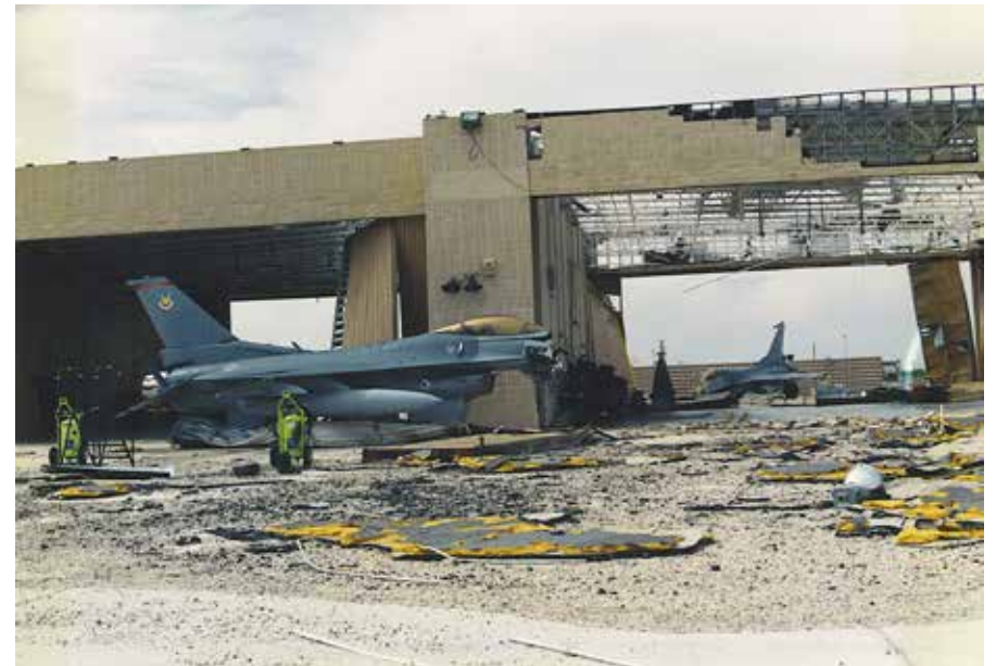
Homestead Air Force Base, post-Andrew damage, 1992.
