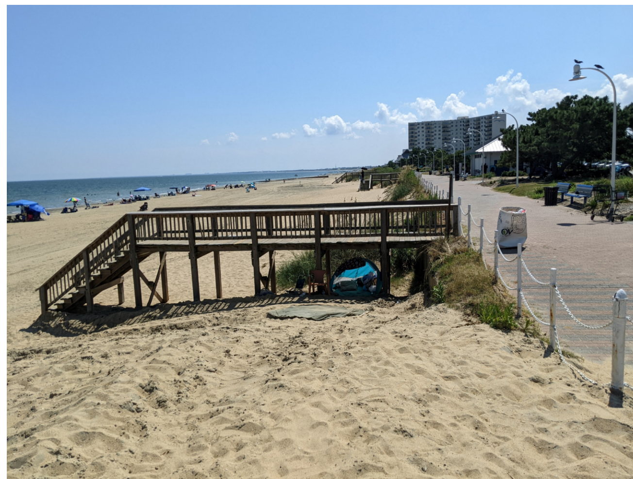
REPLACE WITH ACCESSIBLE ACCESS RAMP
